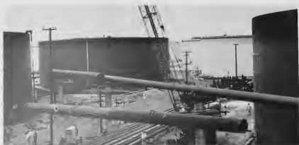
THIS SCENE in the tank farm shows the dimensions of pipe sections as a crane swings them into place. For the longer pieces, two 44-foot sections were welded together before being mounted.
